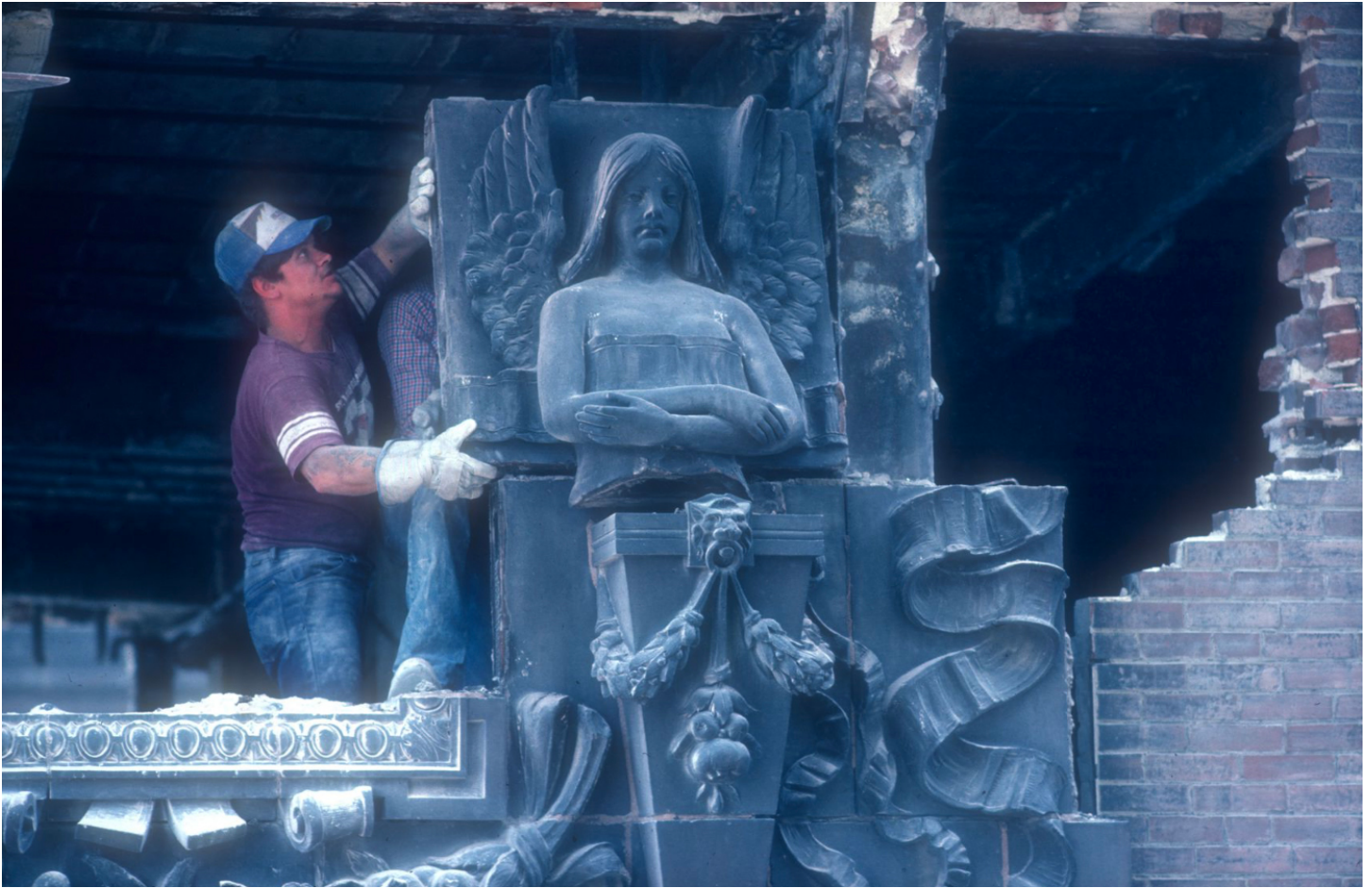
Removing a terra cotta victory figure from the Title Guaranty Building in St. Louis, Missouri, 1983.
